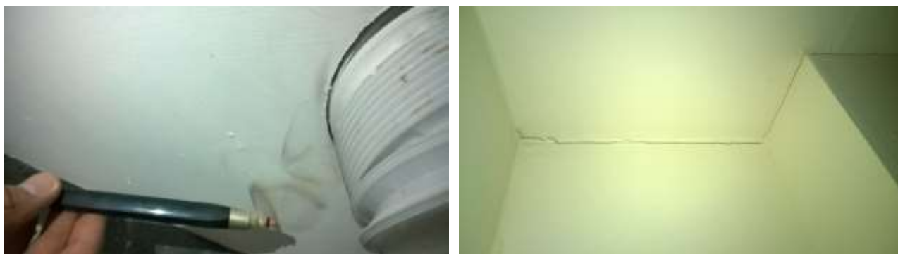
275 Figure 14 (left): leakage around WC discharge pipe. Figure 15 (right): cracks appearing around internal finishes
