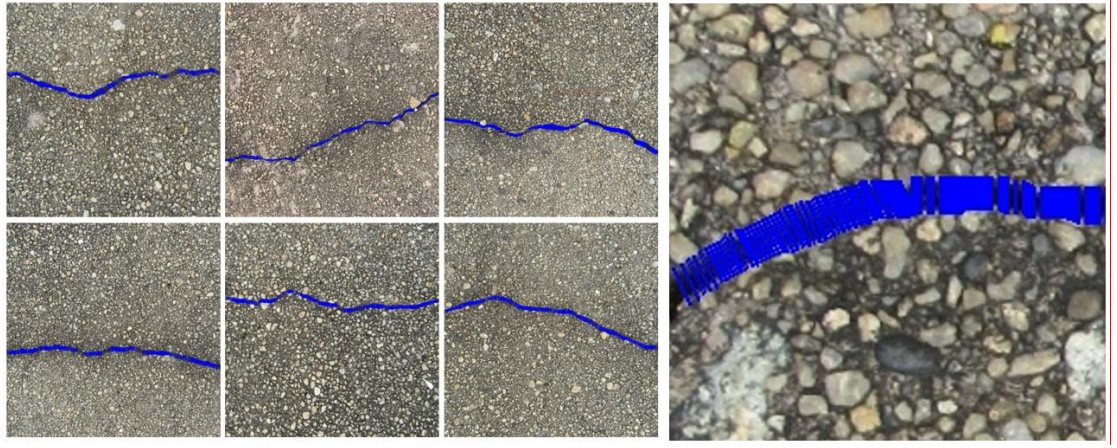
Fig. 9 Measurable point of a section of a crack and its measurement scheme
