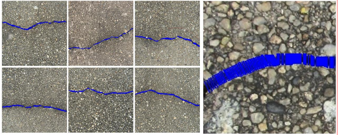
Fig. 9 Measurable point of a section of a crack and its measurement scheme
