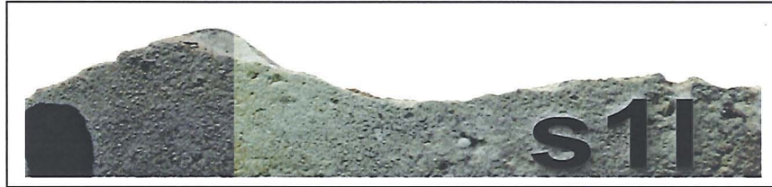
(a) Image of cracked concrete profile.
