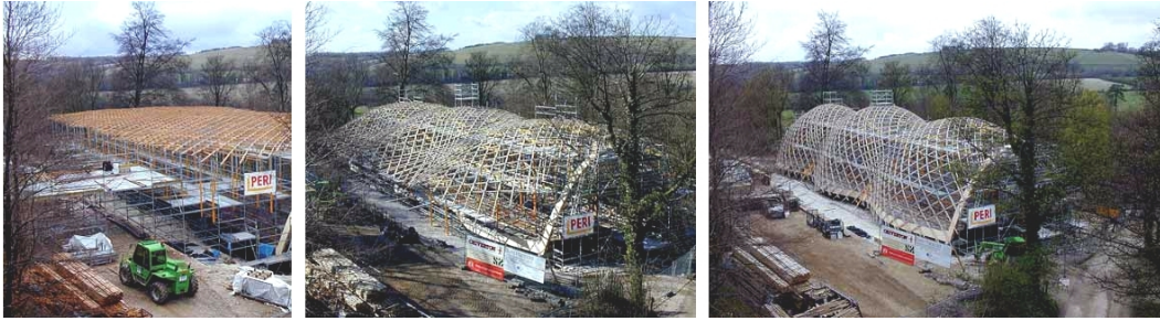
Figure 1.10: Weald and Downland grid-shell, Singleton, Sussex, UK, 2002: Construction phases [Dickson and Harris, 2004].
