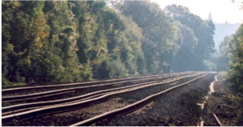
Figure 1.4: Collapse of railway embankment
