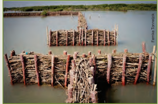
Permeable dams placed to dissipate waves and capture sediments so that mangroves can re-establish themselves and provide erosion protection.
