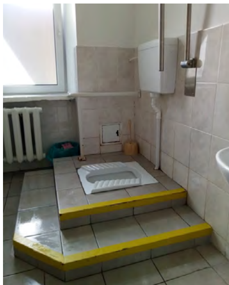
Figure 3: Inaccessible Toilet in the Hospital
