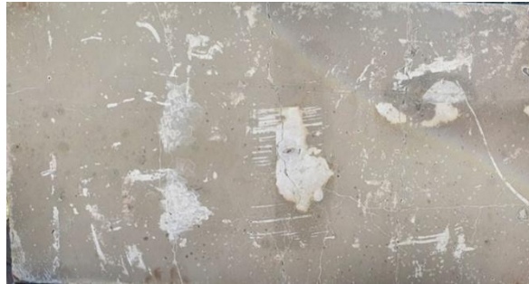
Figure 14b. No major damage with microcracking pattern
