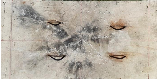
Figure 14a. No major damage with microcracking pattern
