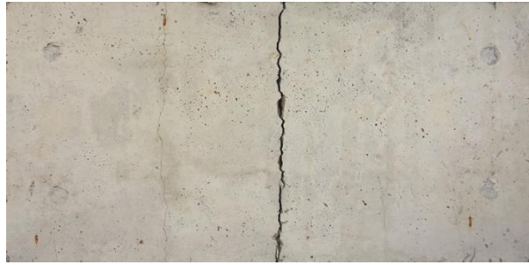
Figure 12b. Complete flexural failure pattern
