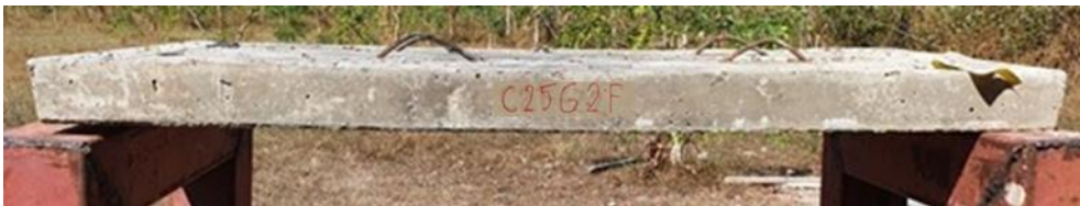
Figure 14c. No major damage with microcracking pattern
