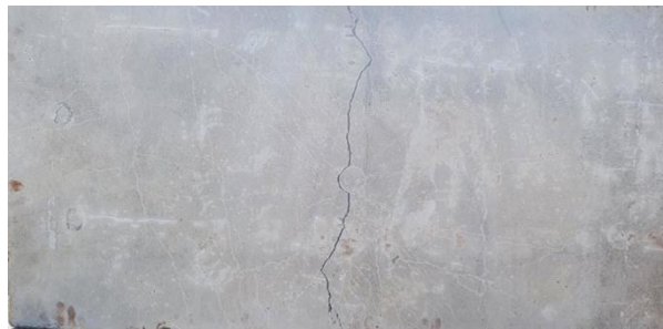
Figure 13b. Flexural cracking pattern
