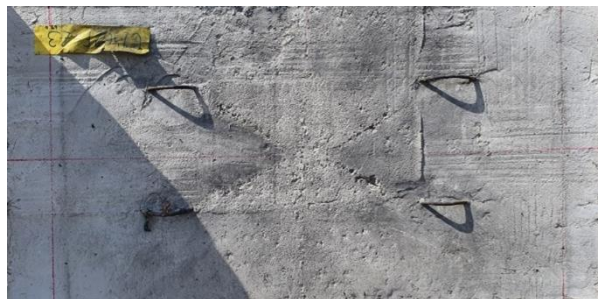
Figure 13a. Flexural cracking pattern
