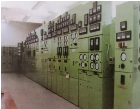
Figure 5b Interior of Marka Power Plant Amman
