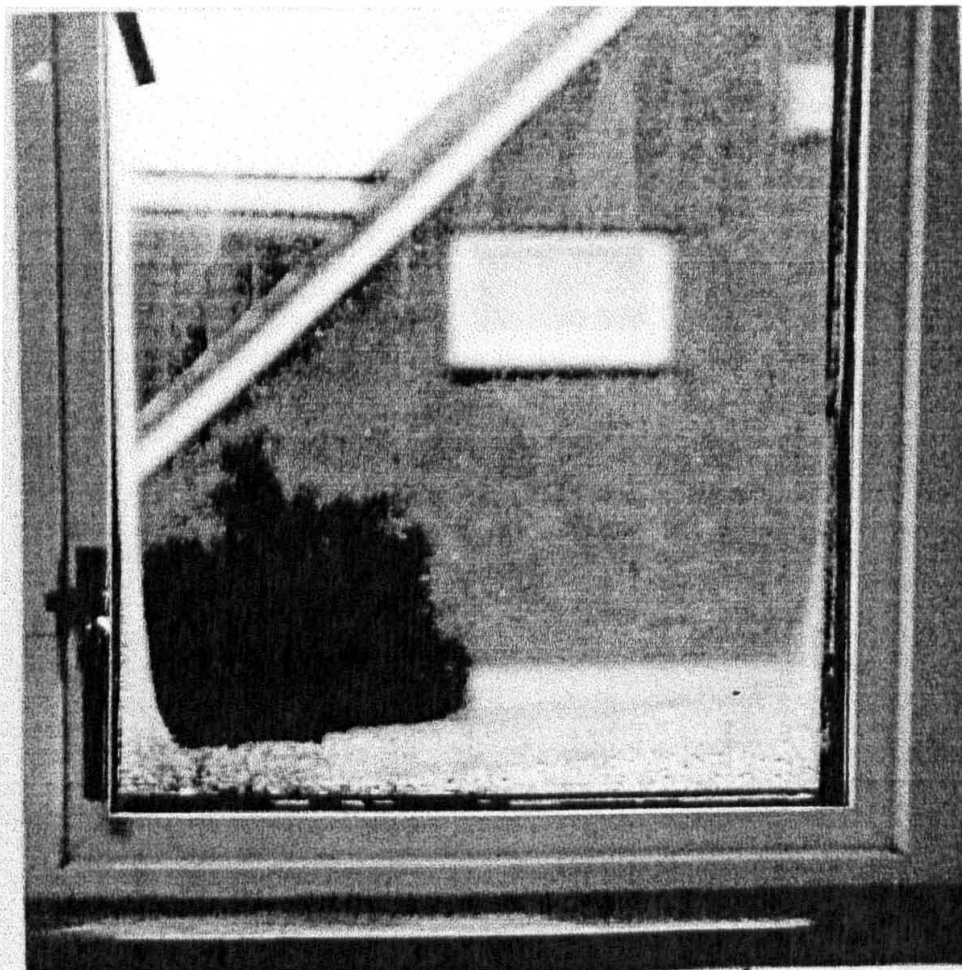
Figure 7.11b Condensation on double glazed window-experimental house (Normal view)
