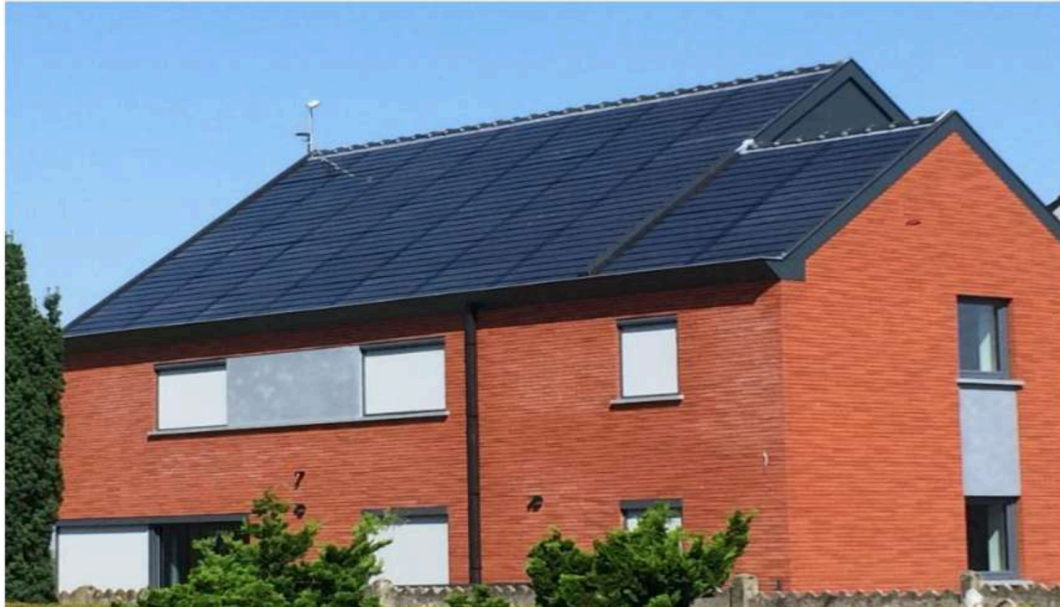
Figure 1: An example of BIPV roofing [10]
