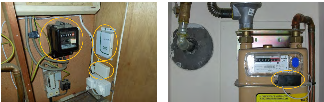
Figure 2.1 - The Ewgeco energy logger connected to electricity (left) and gas (right) meters. Logging equipment circled.
