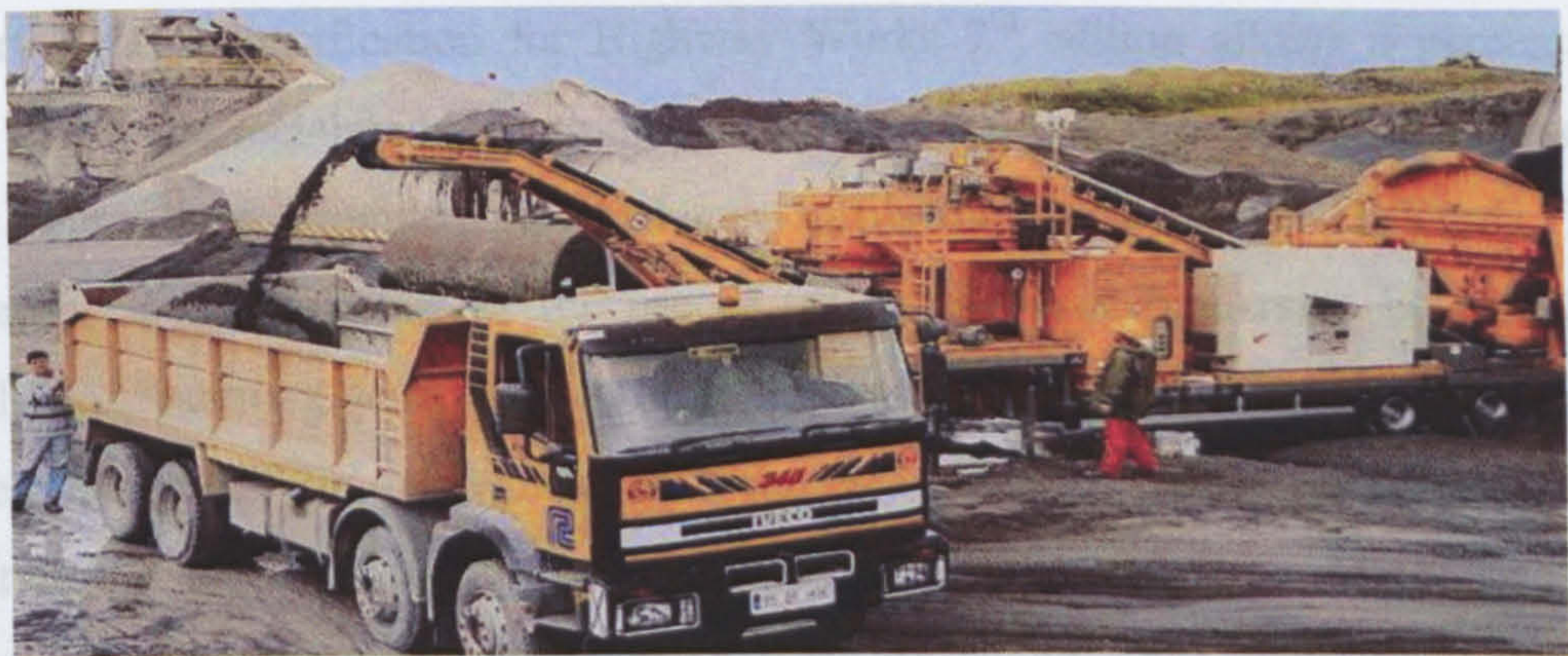
Fig. 2.22 - Portable cold mix plant used to make foamix (Wrigten 2000)
