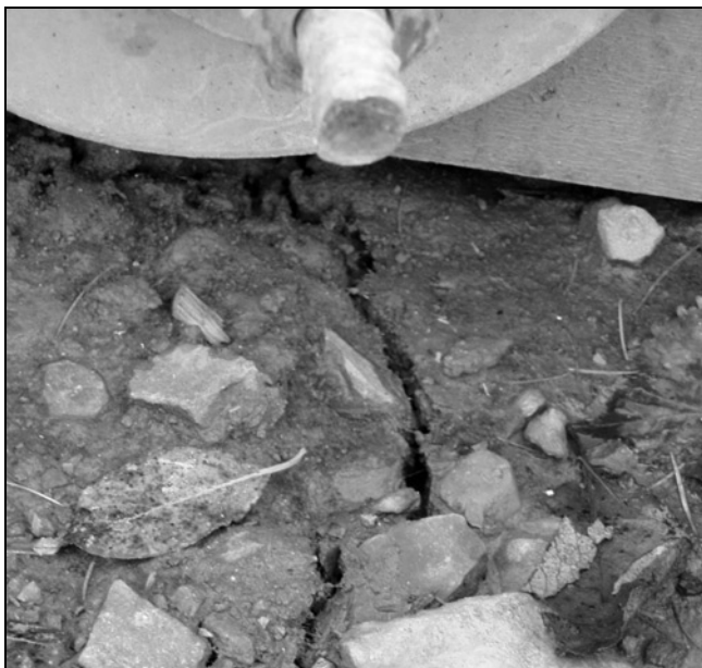
Fig. 8. Bridge at Glentress: effect of foundation slip (crack opening near a support) under the full quarter-point loading
