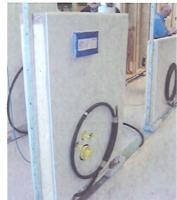
c) Toilet panel
