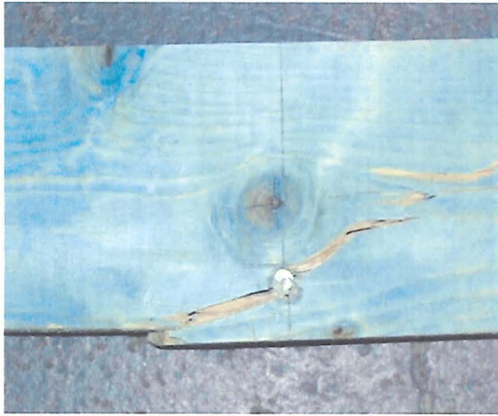
a) Split propagating from an area of high stress concentration in the bottom chord
