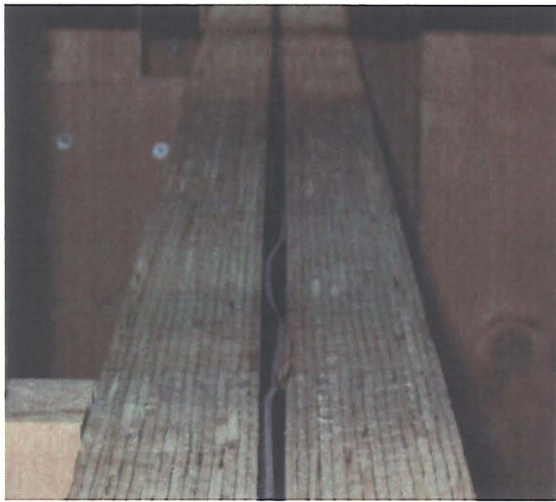
c) Buckling of steel in the top chord of an LVL fitch beam
