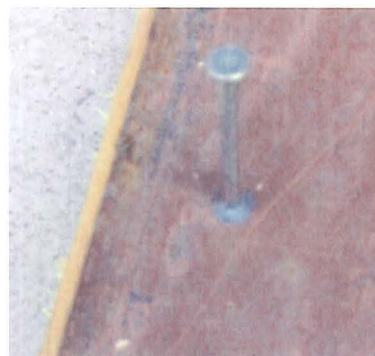
b) Headside of nail after removal of timber showing cold weld
