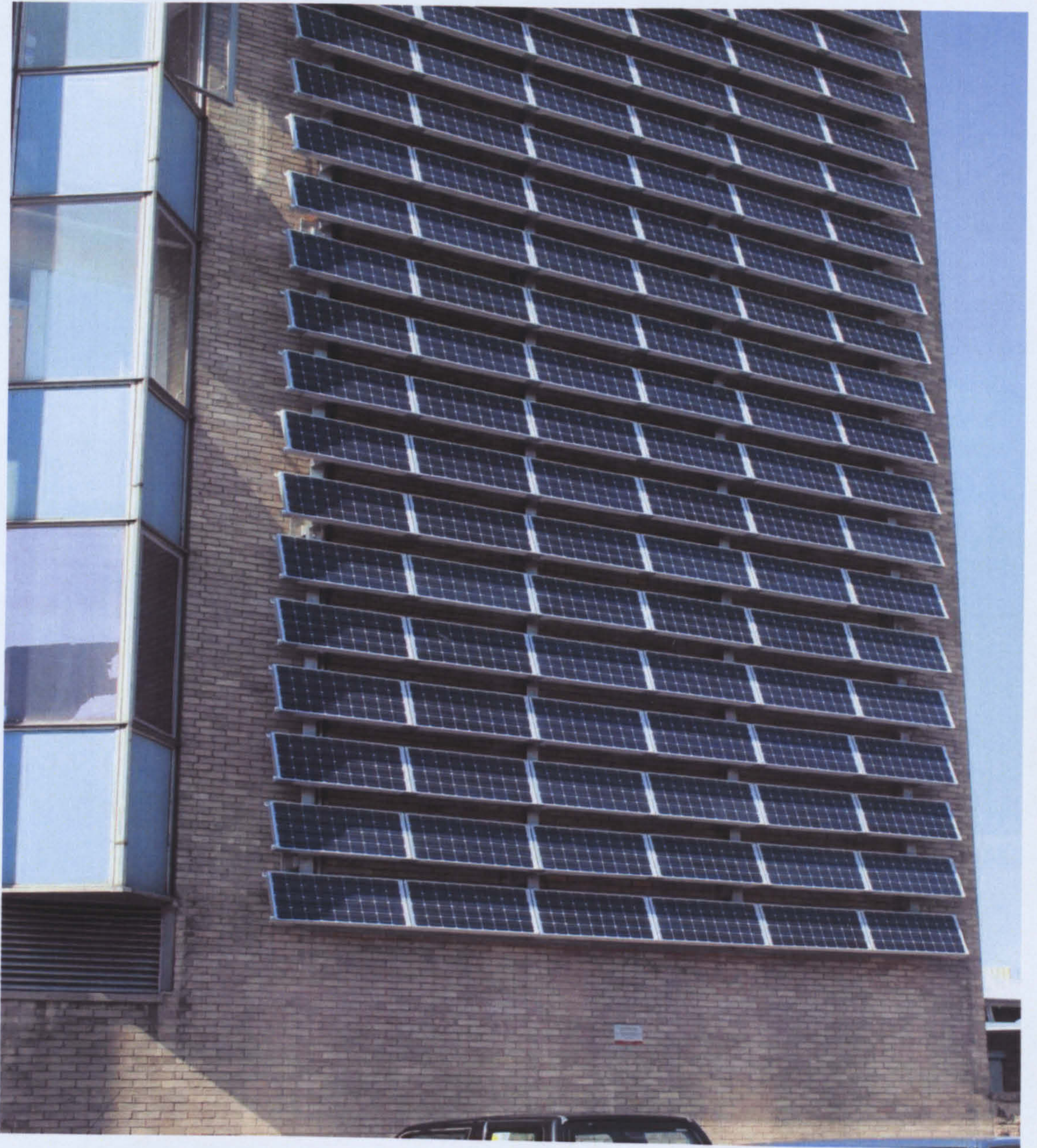
Figure 2.3.2.2 Napier PV facade experiencing shading from protruding bay window in the afternoon (08/05/06 at 3:45 PM).
