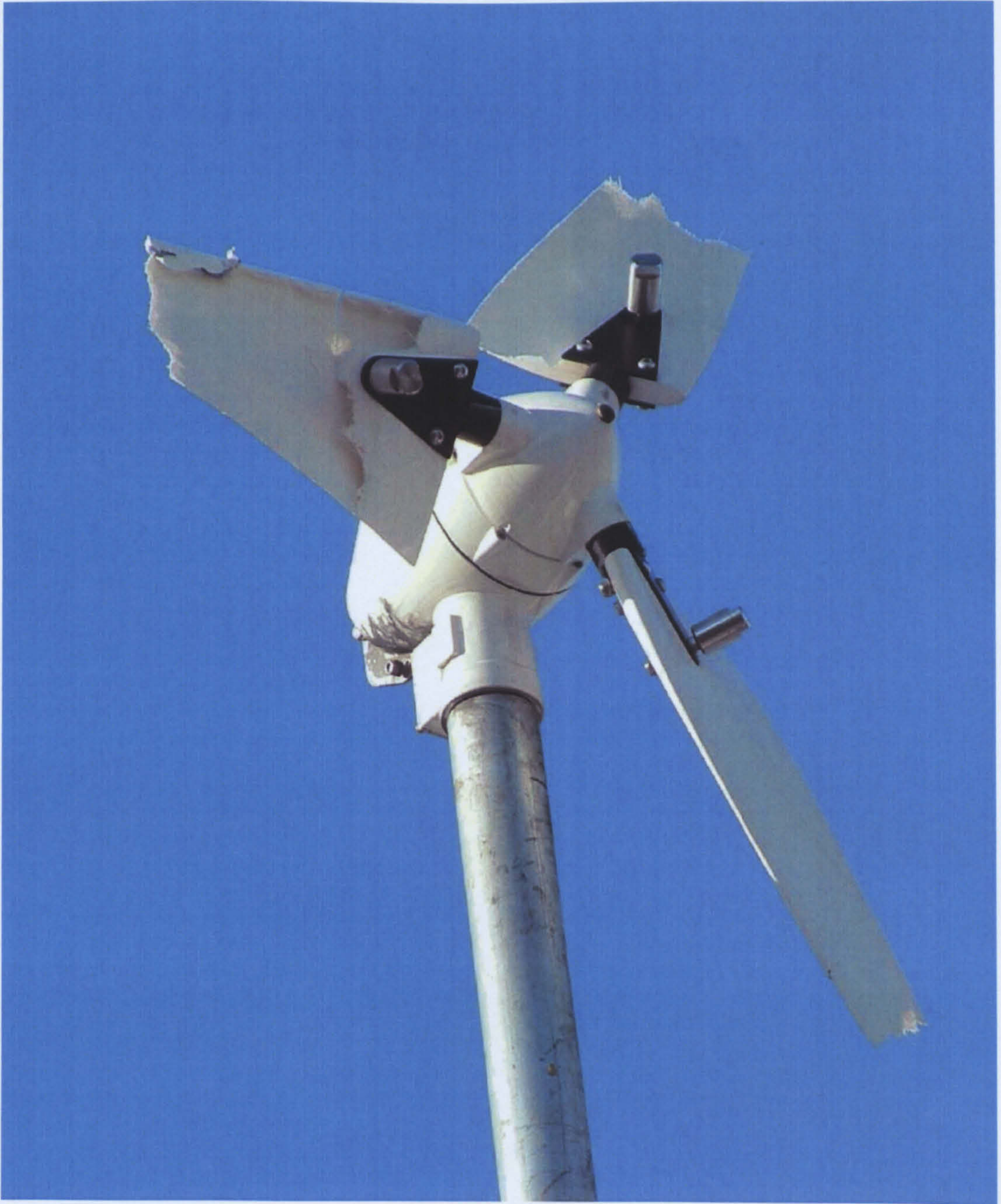
Figure 6.2.2.2 Ampair 600 turbine shown with broken blades and loss of tail fin (February 2008).
