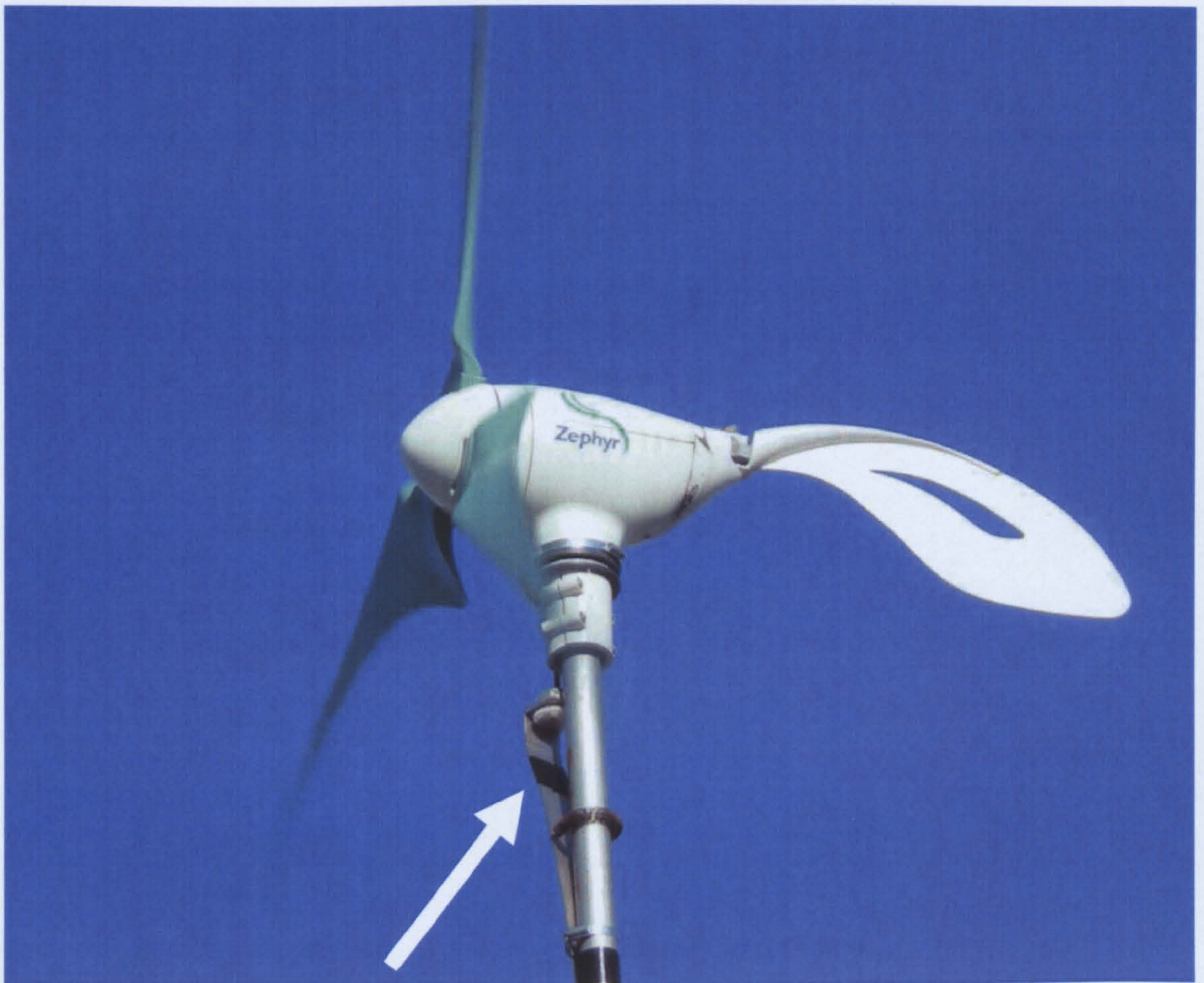
Figure 2.22.1.1 Wind turbine direction indicator installed on Airdolphin turbine (Edinburgh Napier University)
