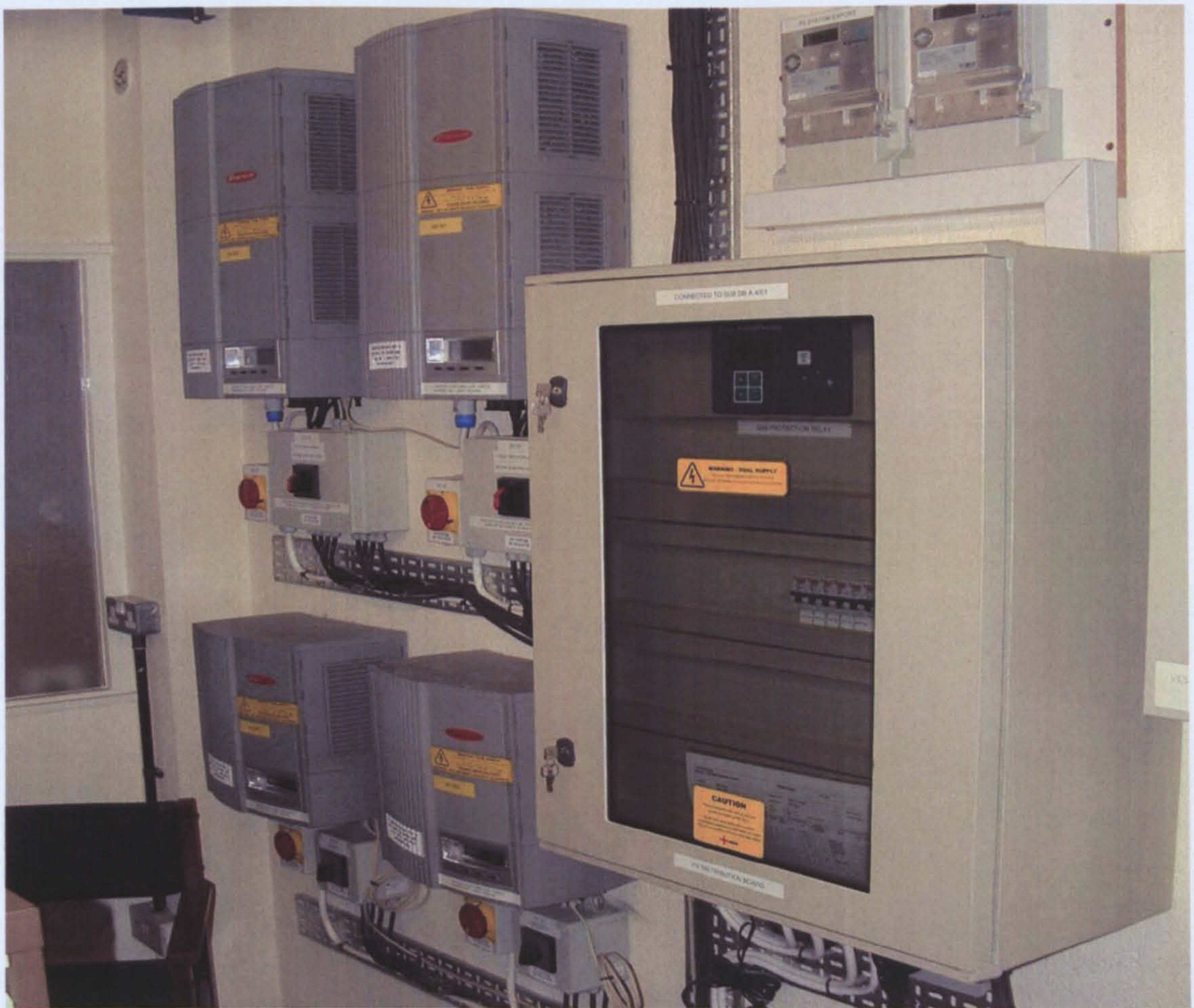
Figure 2.3.2 Napier PV facade control board.
