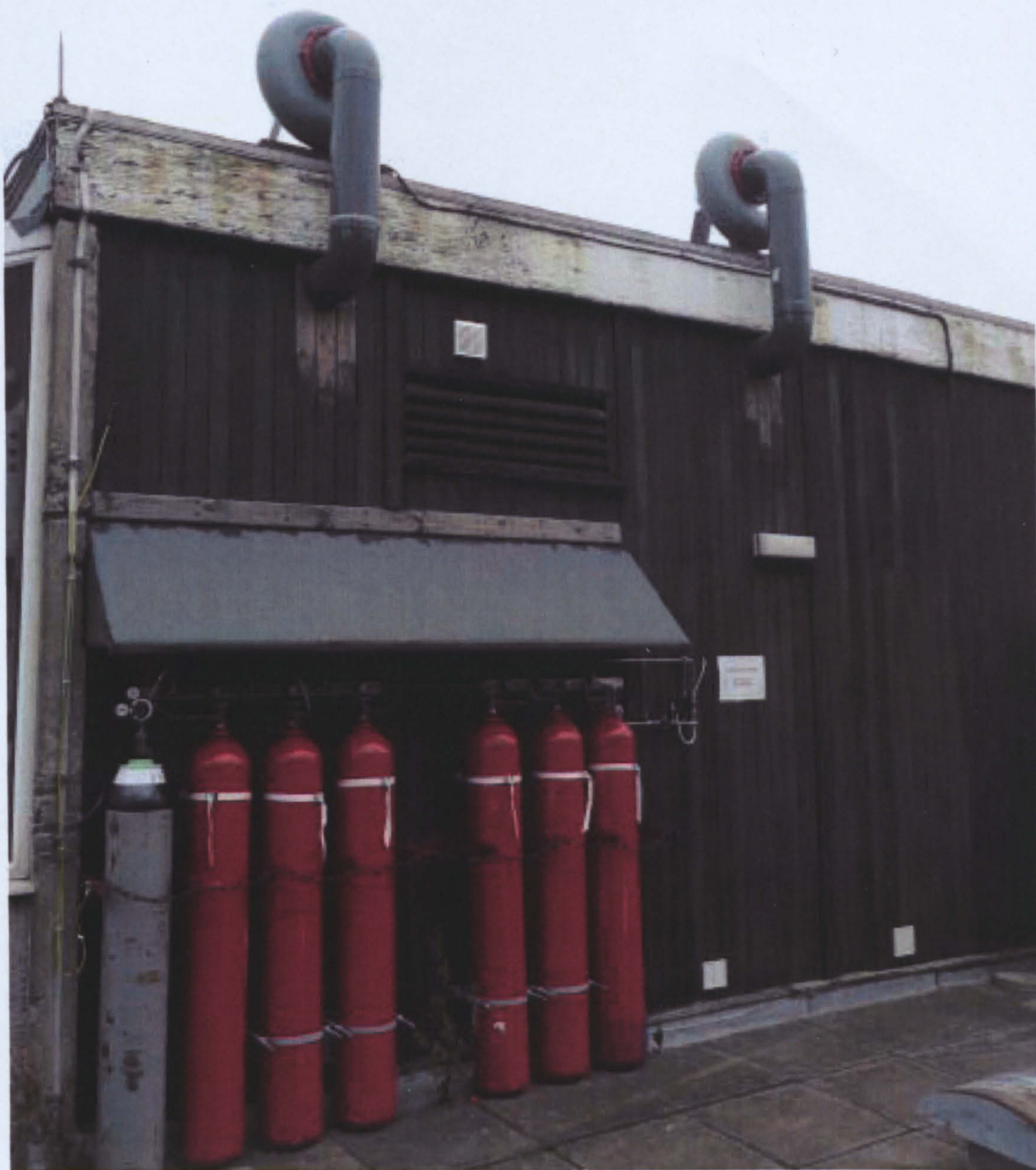
Figure A.11.1 Gas storage cylinder bank located on the University's roof behind the hydrogen lab. Note one nitrogen cylinder and 6 red hydrogen cylinders. Two high-level extraction fans can also be seen on the lab's roof.
