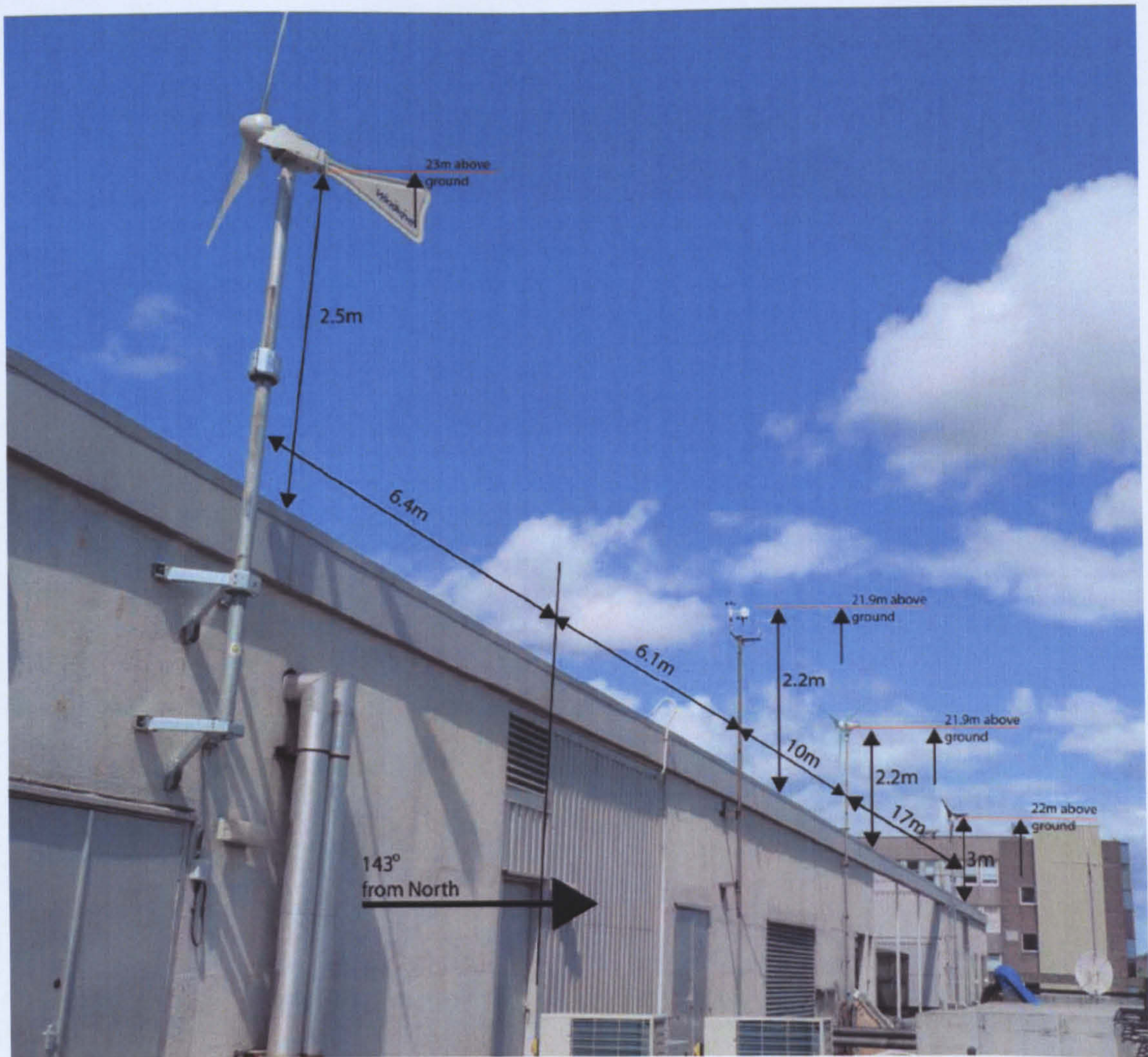
Figure 6.2.2. Edinburgh Napier University Merchiston Campus rooftop test site. (From the left, Windsave turbine, wind monitoring station, Airdolphin turbine, Ampair 600 turbine and anemometer).
