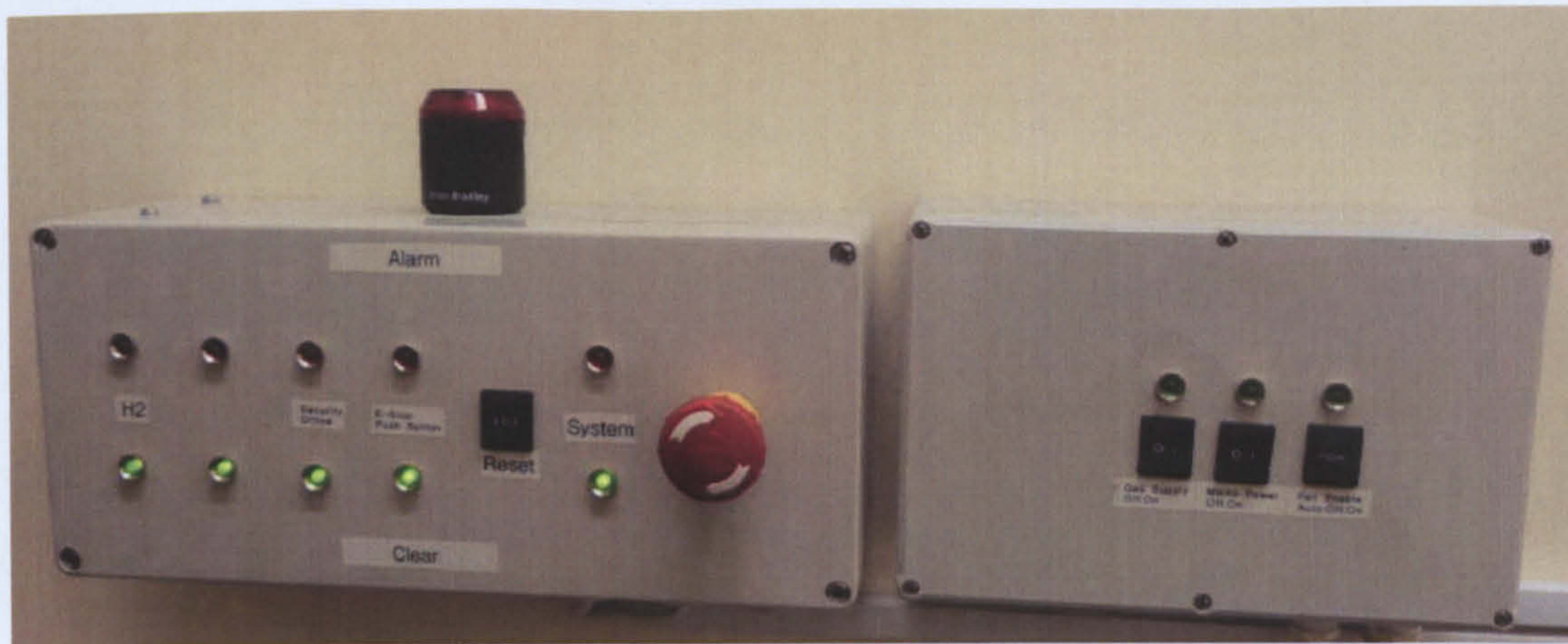
Figure A.15.8 Hydrogen alarm and control panel.
