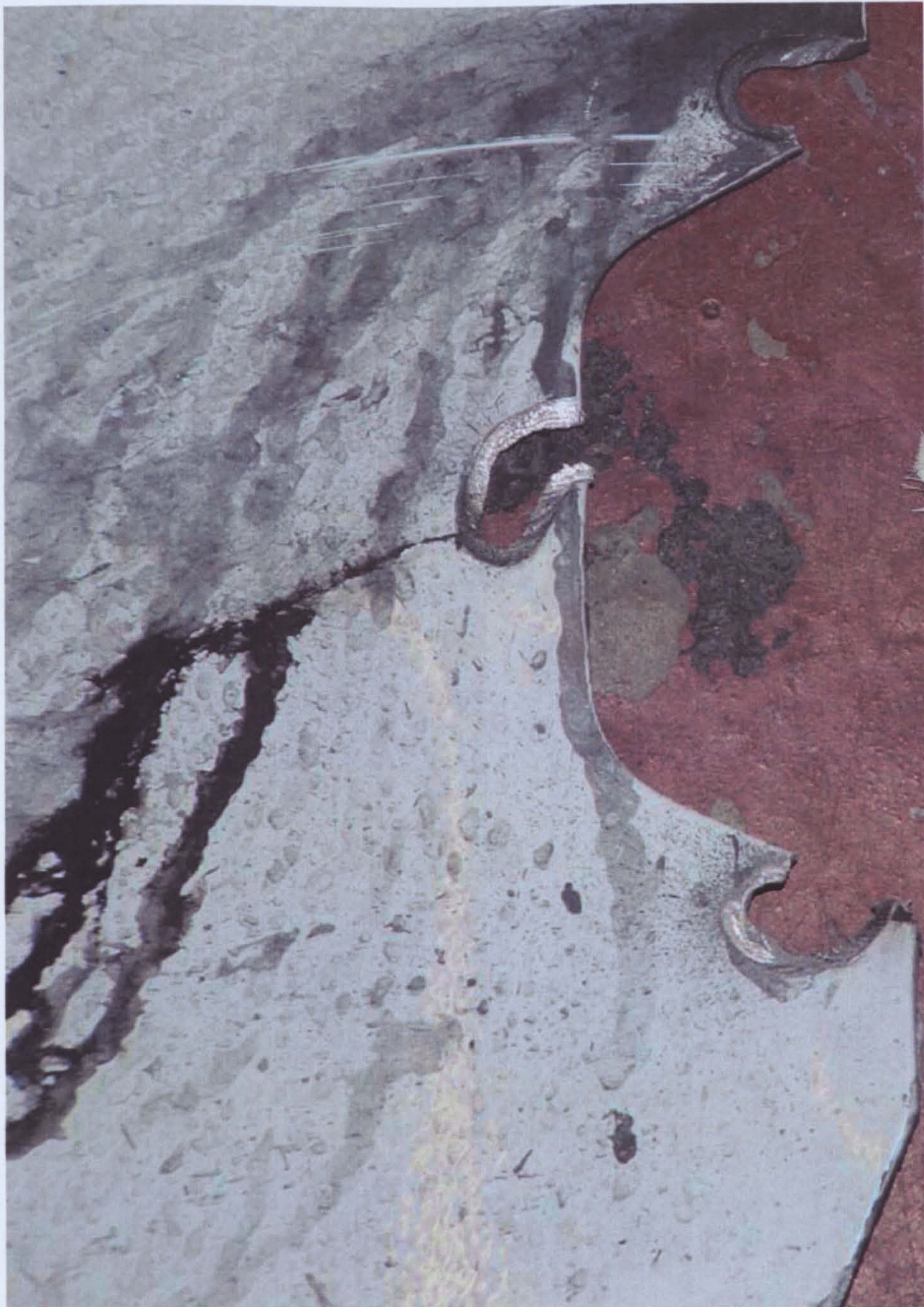
Figure 6.2.2.3 Broken Ampair 600 tail fin (failed due to fatigue, February 2008).
