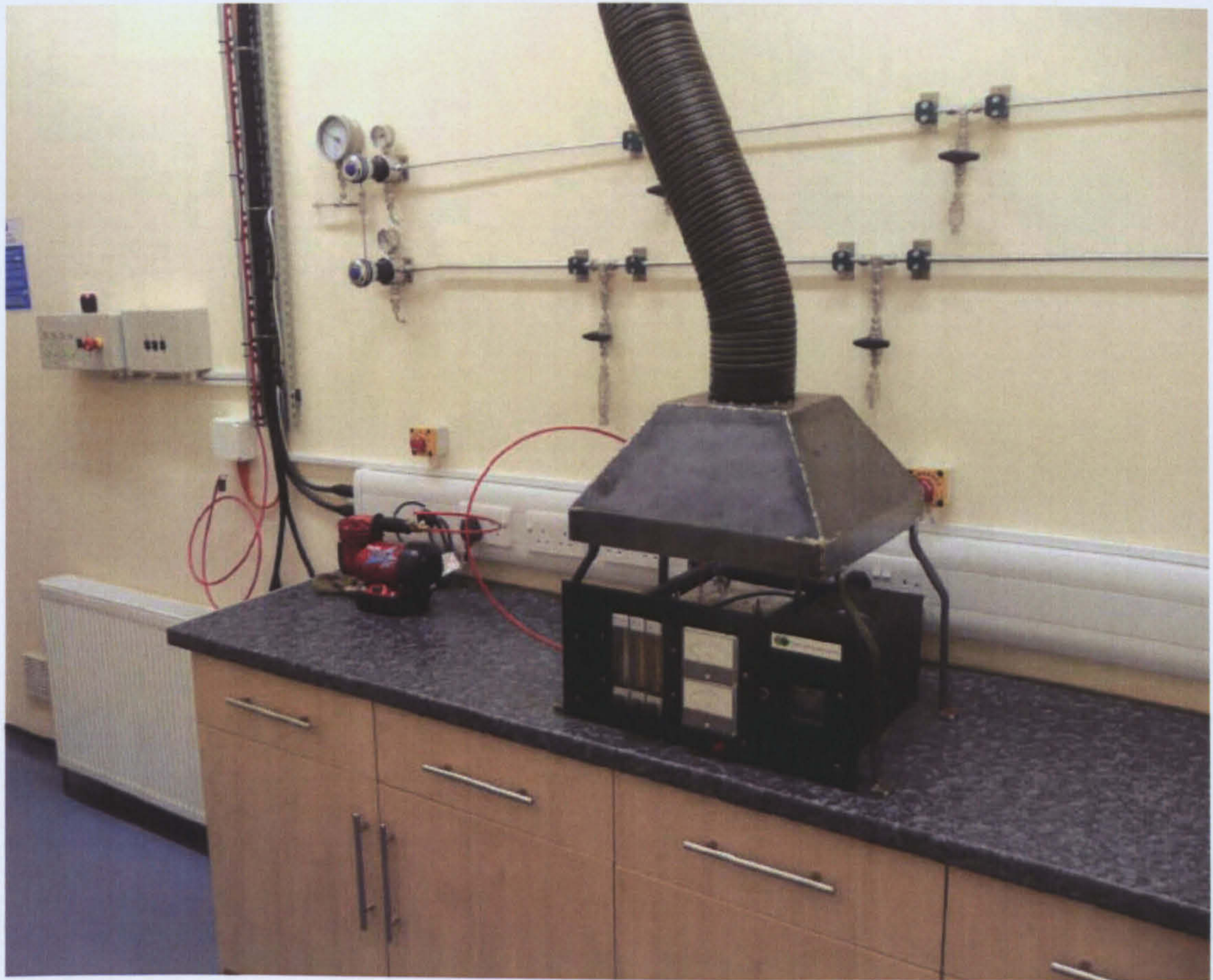
Figure A.15.2 Second view of hydrogen research laboratory, note hydrogen alarm safety system on left-hand side.
