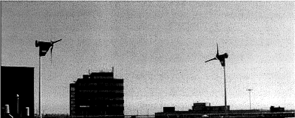
Figure 5.19 Two Proven WT6000 turbines installed on the roof of Kirklees city council building
