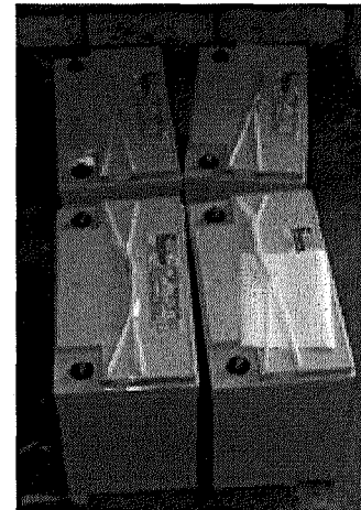
Figure3.5: The batteries bank used in Napier stand-alone system
