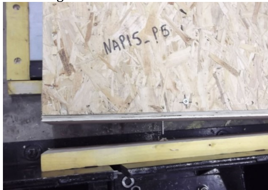
Sheathing failure observed in P15-P16
