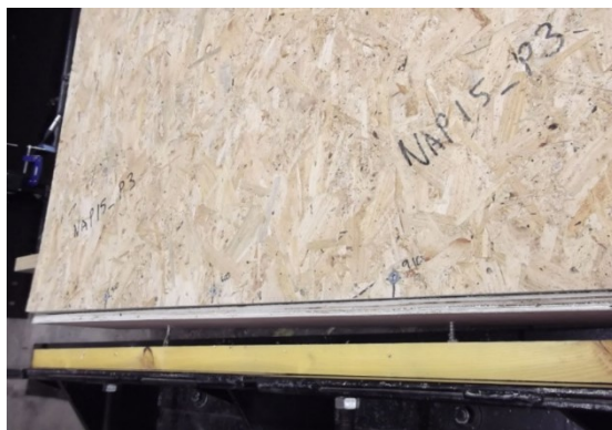
Sheathing failure observed in P13-P14
