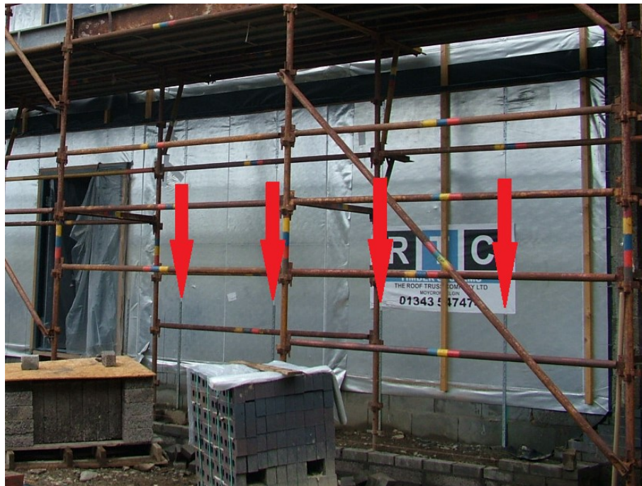
Figure 4-27 Timber frame closed panel secured to substrate by holding down straps only at every other stud.
