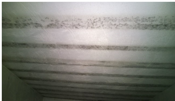
a) Concrete joist on a roof. Mould growing as a consequence of linear thermal bridge
